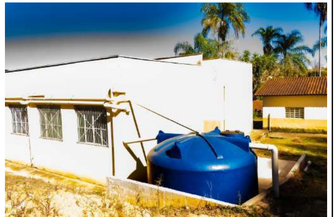
Figure 22: Inconfidentes Campus rainwater recovery system.
