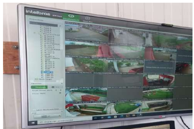
Figure 4: Pouso Alegre Campus CCTV.
