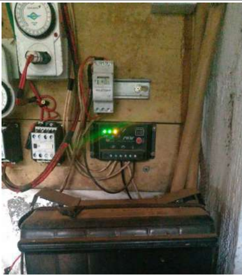
Figure 27: Machado Campus hydroponic photovoltaic system.
