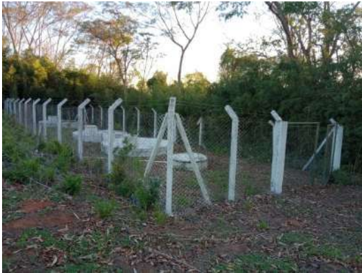
Figure 13: Machado Campus sewage treatment system with septic tank, anaerobic filter and sink.
