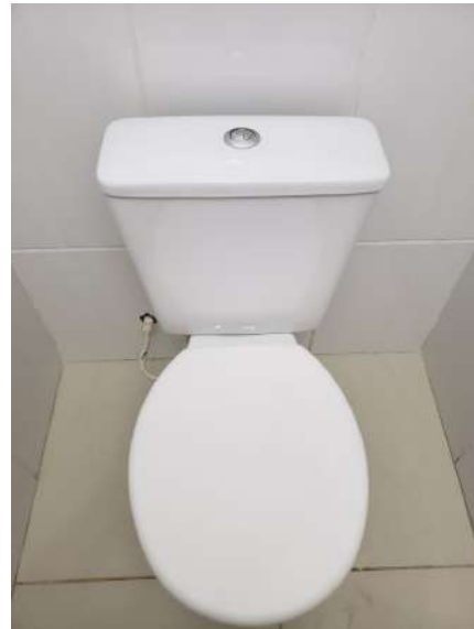
Figure 10: Rectory toilet flushing with double activation.
