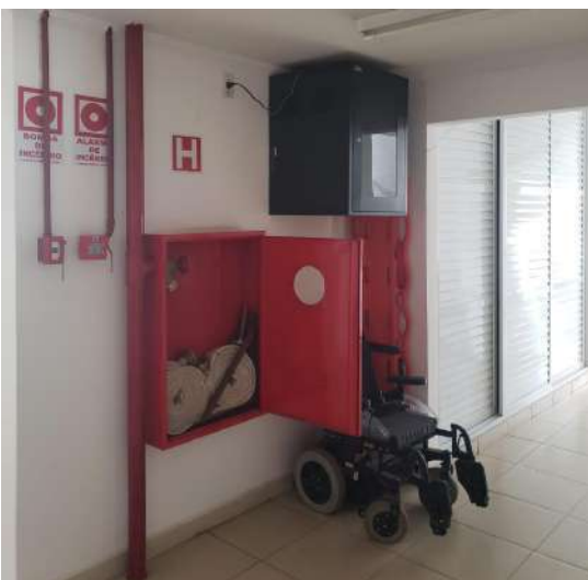
Figure 9: Rectory fire alarm and hydrant.
