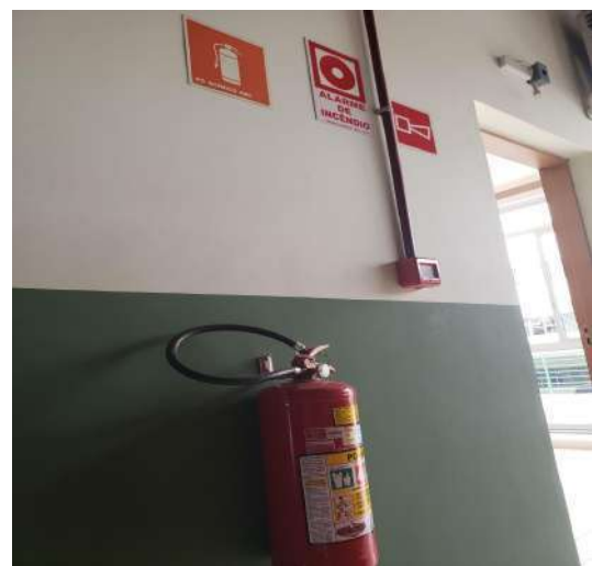
Figure 10: Rectory fire alarm and fire extinguisher.
