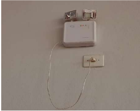
Figure 5: Pouso Alegre Campus emergency lights.
