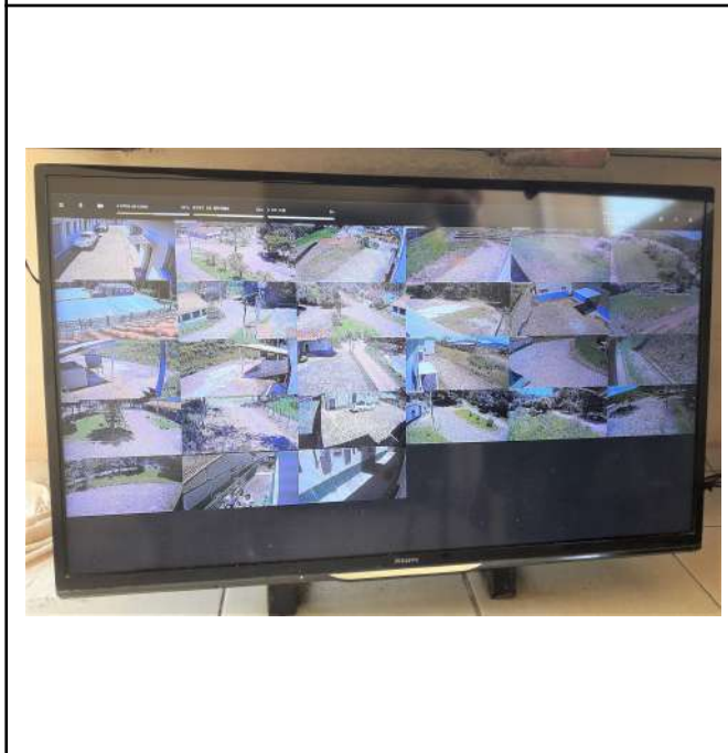
Figure 13: Inconfidentes Campus CCTV.
