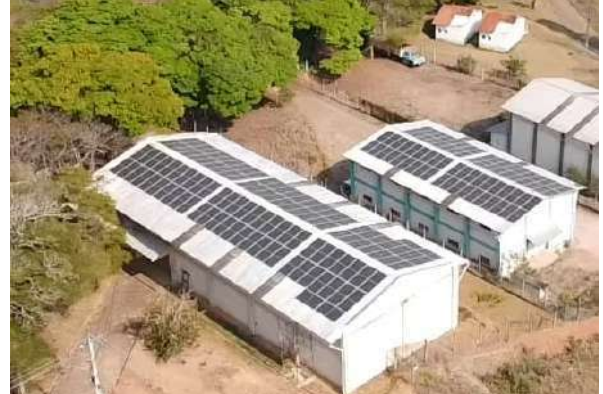
Figure 22: Machado Campus implementation of new photovoltaic modules.
