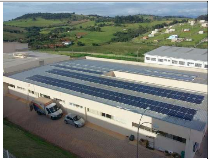
Figure 6: Campus Pouso Alegre solar power plant.
