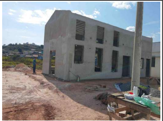
Figure 28: Construction of the new Chemical Warehouse at the Poços de Caldas Campus.
