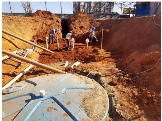
Figure 20: Machado Campus implementation of the Sewage treatment system of the Coffee Center of Excellence.
