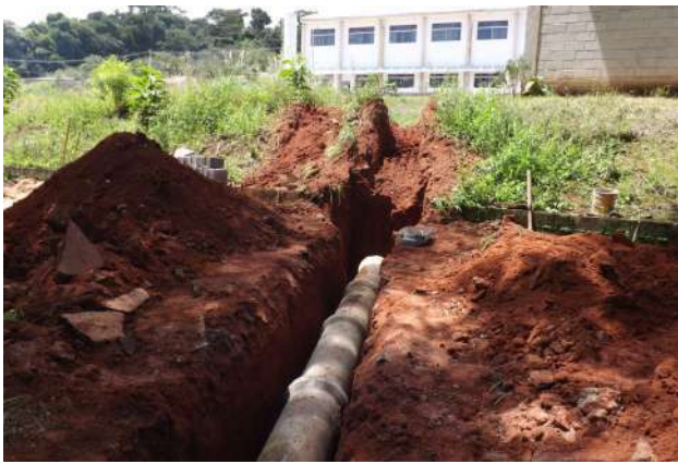
Figure 7: Machado Campus streets drainage.
