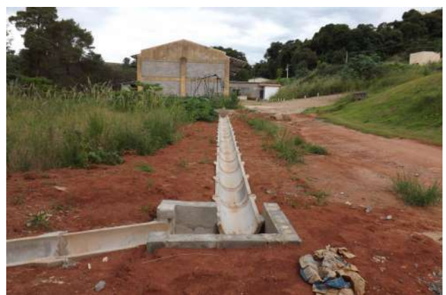
Figure 8: Machado Campus streets drainage.
