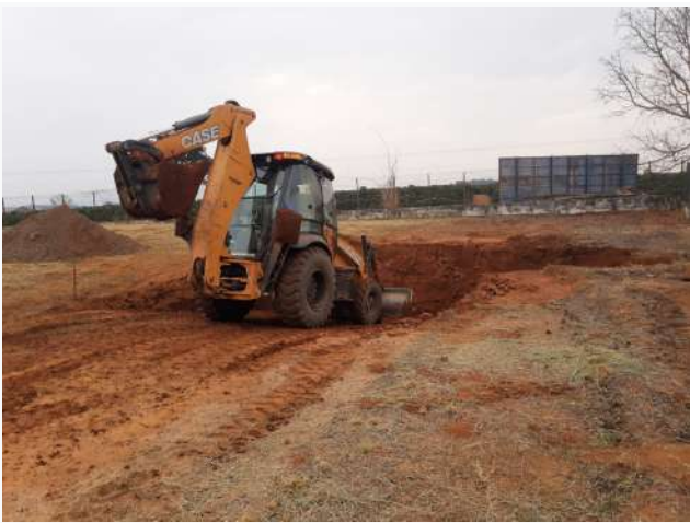
Figure 19: Machado Campus implementation of the Sewage treatment system of the Coffee Center of Excellence.
