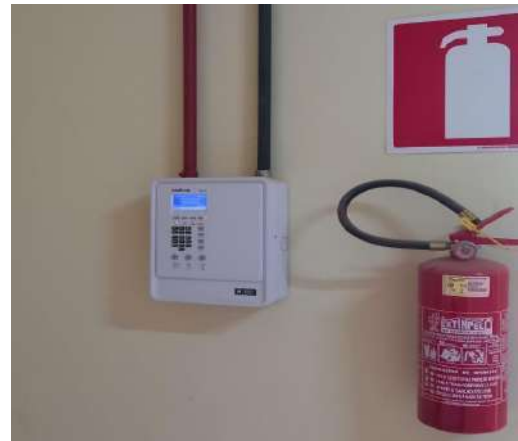
Figure 8: Pouso Alegre fire alarm and fire extinguisher.
