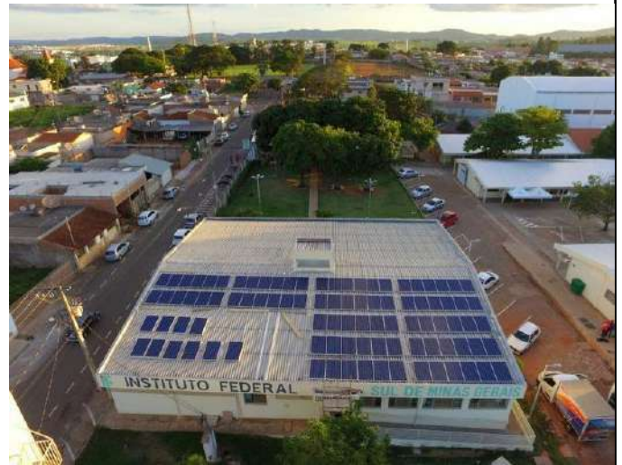
Figure 4: Campus Passos solar power plant.
