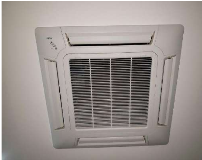
Figure 7: Rectory efficient air conditioning.
