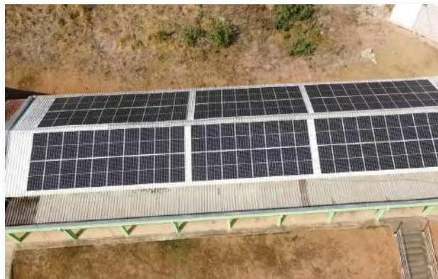
Figure 21: Machado Campus implementation of new photovoltaic modules.
