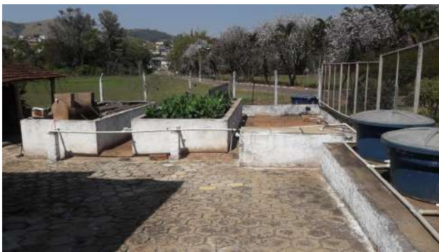
Figure 7: Figure 16: Inconfidentes Campus Wetland System installed in the dairy sector.
