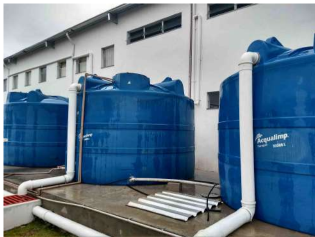
Figure 9: Poços de Caldas Campus rainwater reservoir tanks.
