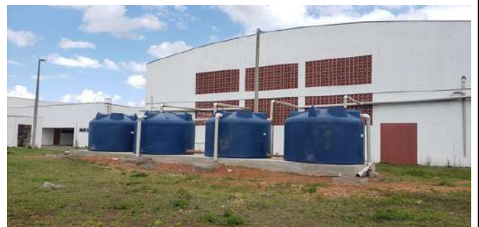
Figure 20: Poços de Caldas Campus rainwater reservoir tanks.
