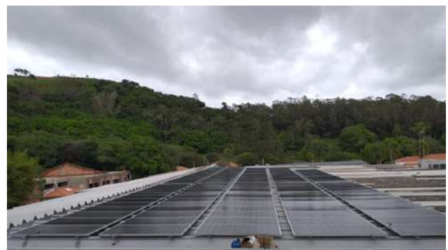
Figure 40: Carmo de Minas Campus new photovoltaic panels in the auditorium.
