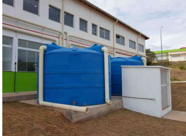
Figure 10: Pouso Alegre Campus rainwater reservoir tanks.
