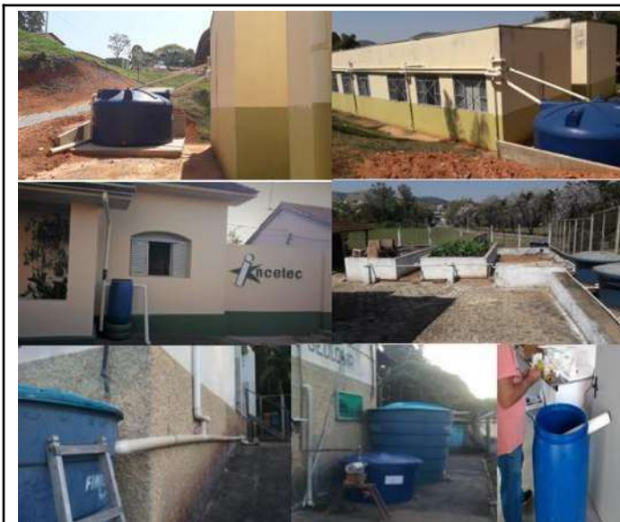
Figure 1: Campus Inconfidentes rain harvesting system.
