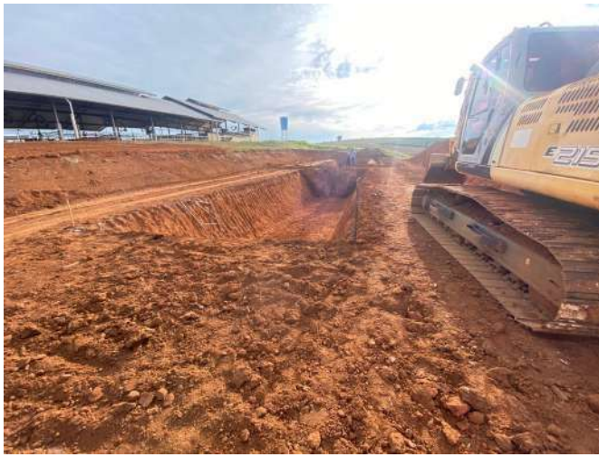
Figure 21: Construction of a new rainwater reservoir with a capacity of 500 thousand liters on the Muzambinho Campus.
