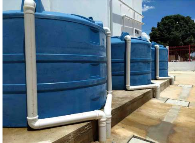
Figure 8: Passos Campus rainwater reservoir tanks.
