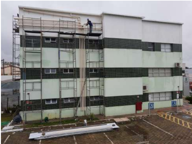
Figure 19: Rectory new rain harvesting system.
