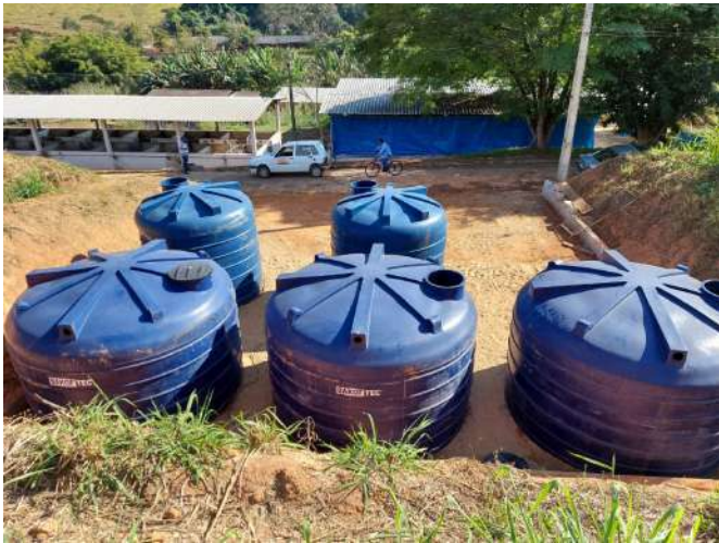
Figure 17: Machado Campus new rainwater reservoir tanks.
