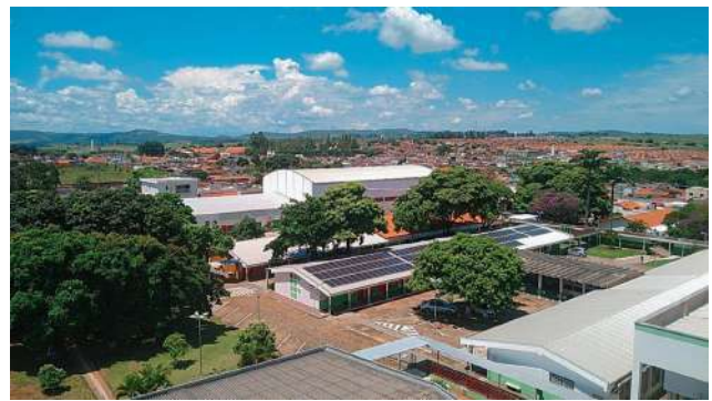
Figure 6: Passos Campus new photovoltaic panels.
