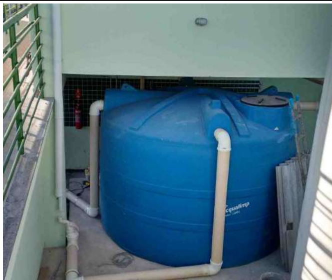
Figure 11: Rectory rainwater reservoir tank.
