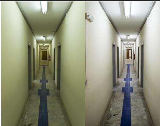
Figure 9: Campus Inconfidentes previous lighting compared to new LED lighting.
