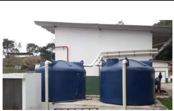
Figure 24: Carmo de Minas Campus rainwater catchment system
