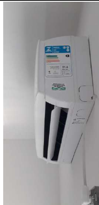
Figure 6: Campus Carmo de Minas efficient air conditioning.
