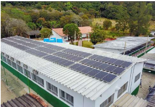
Figure 3: Carmo de Minas Campus photovoltaic panels for solar energy production through the IF Solar Program .
