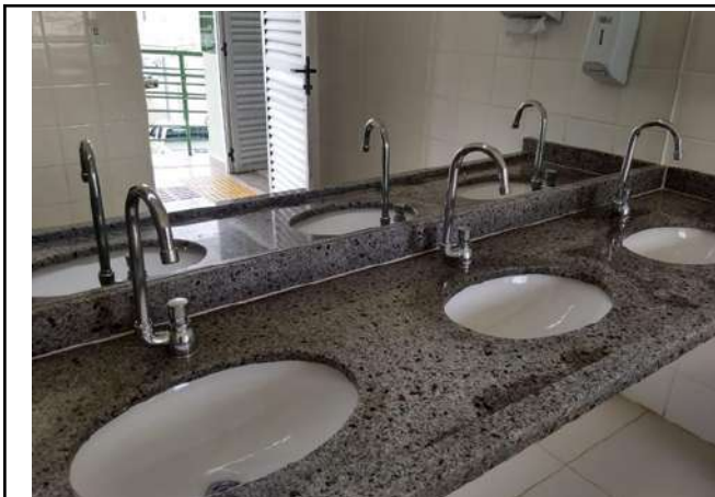
Figure 1: Rectory time delay water taps.
