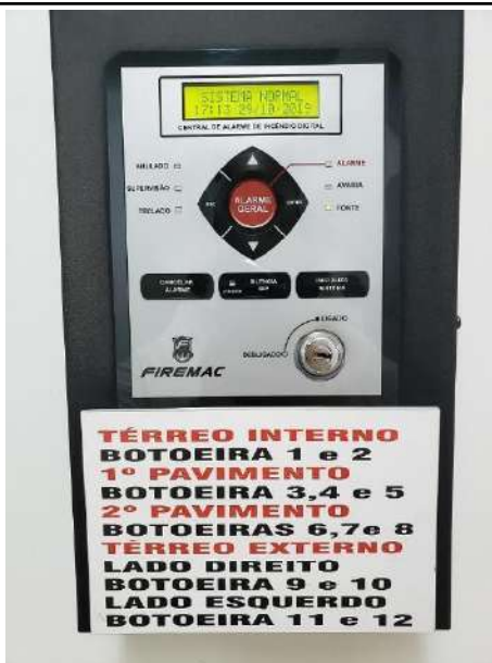
Figure 3: Rectory fire-fighting system – Fire alarm.
