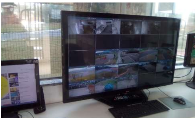
Figure 3: Machado Campus CCTV in entrance.
