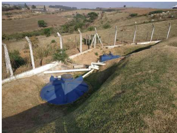
Figure 7: Muzambinho Campus rainwater reservoir tanks.
