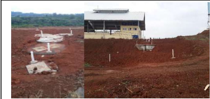
Figure 5: Muzambinho Campus waste treatment.
