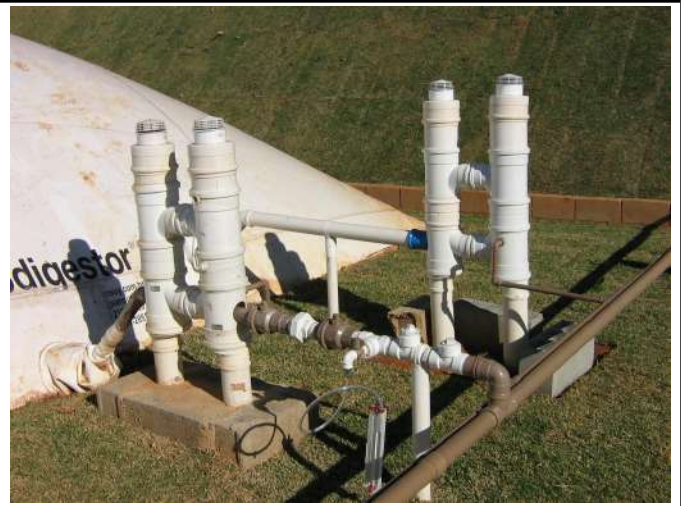
Figure 14. Swine waste treatment unit for biogas production.
