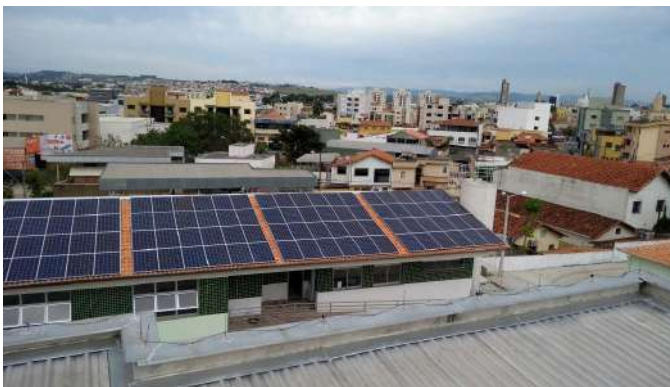
Figure 9: Rectory solar power plant.
